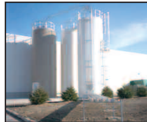
Material is separated from the airstream by a cyclone or filter receiver. Material drops through a rotary airlock and is conveyed by pressure to a takeoff into a silo.
