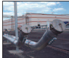
A railcar manifold aids the removal of material from the railcar into bulk storage silos.
