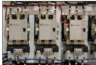
Close-up of the inside electrical panel
