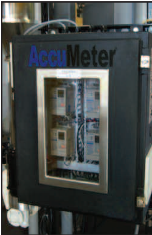
Motor Drive Panel
